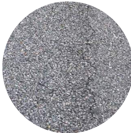
Unreinforced section with cracking
